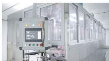
Cell Automatic Cleaning Line
